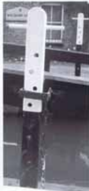
One of the original 'peg-and-hole' paddles at Walsham Gates. Most of the other locks on the Navigation have been converted to the more conventional 'rack and pinion' gear.
