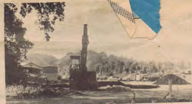
● The heavy machinery moves in and roads begin to take shape. This view of the Goldsworth Park development site was taken from Arthur's Bridge Road.
